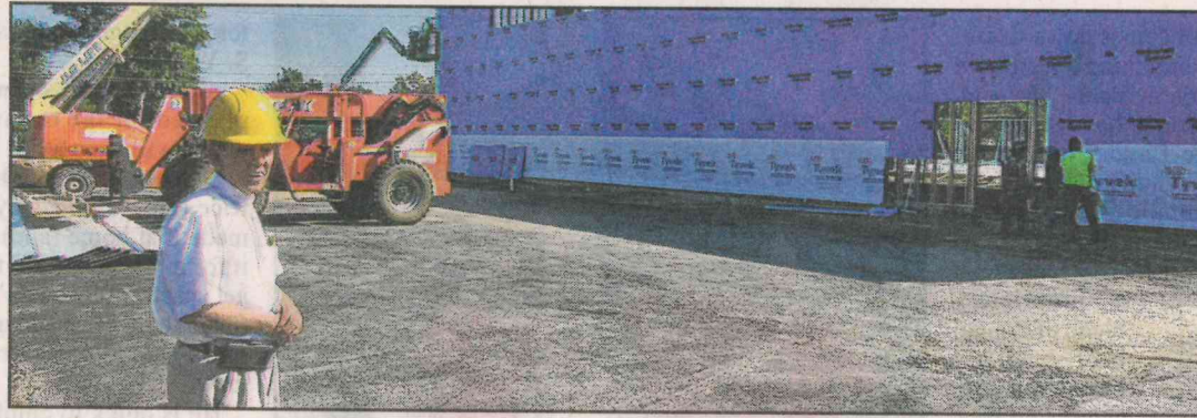
The Rev. Keung Lee, senior minister at the Korean Church of Columbus at 2825 Snouffer Road, surveys progress on a building that would provide additional space for youth programs and worship services. The $2 million project is expected to be completed by the end of the year.
